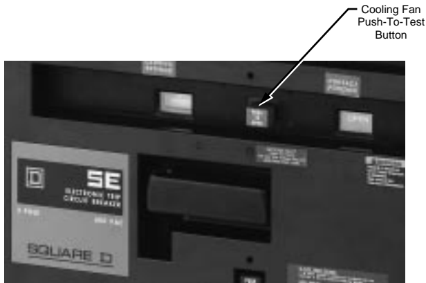
SE Cooling Fan Push-To-Test Feature
