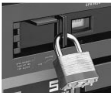
Padlocked Drawout Mechanism
