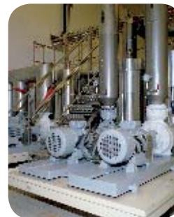
Pumps, compressors, fans
